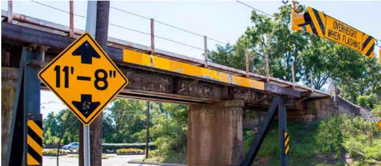
Figure 122: Low Bridge Clearance Signage
