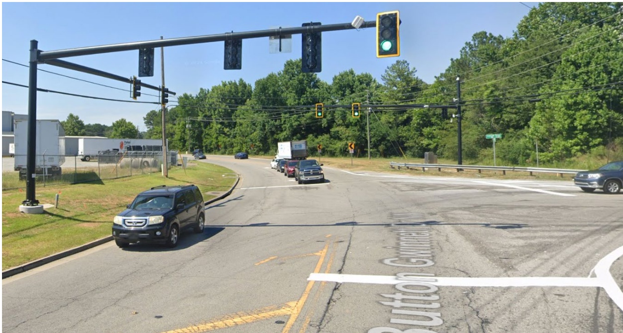
Figure 13: Supplemental Signal Head on Right Supported by Mast Arm
