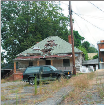
This historic "Ingleside" home on Maple Street is falling apart
