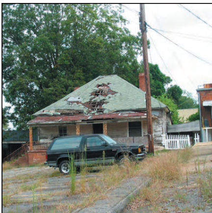
Deteriorated house on Maple Street
