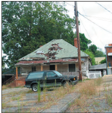
This Maple Street home is in Dilapidated condition
