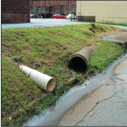
Storm drains empty directly into Center Street and suggest that the public realm is a dumping ground
